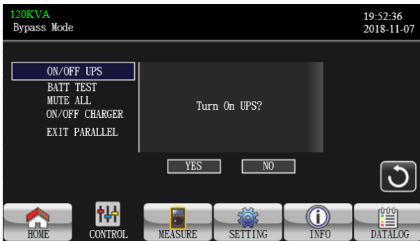
TURN ON UPS
